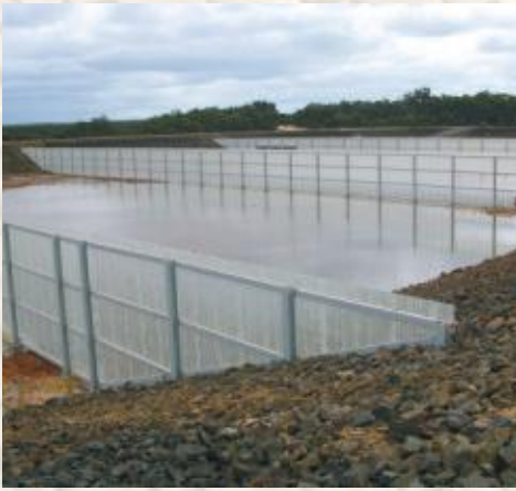
Webglas GC+ – Sewage Treatment Plant, Anglesea, VIC
